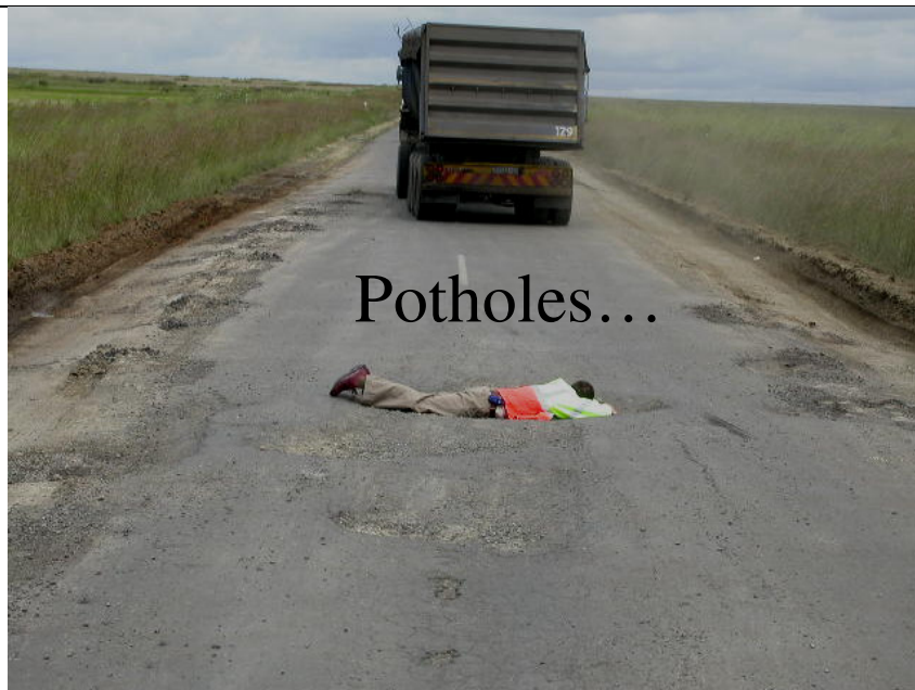
Figure 2: Failure of a secondary provincial road in Mpumalanga, not designed to carry this type of traffic.
